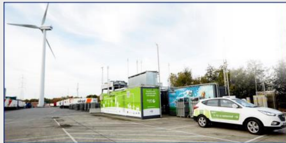
Colruyt Group, Halle (Electrolysis +RE)
