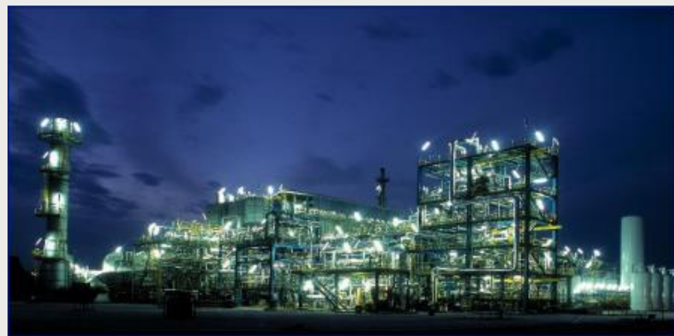
Air Liquide, Port Jerome (SMR +CCS)
